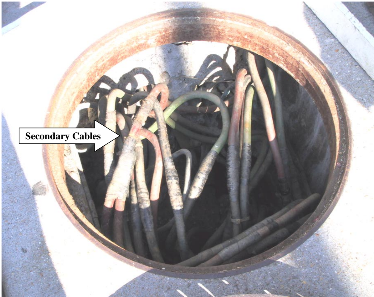
Figure 5 Manhole (Handhole) in Georgetown Crowded with Secondary Cables
