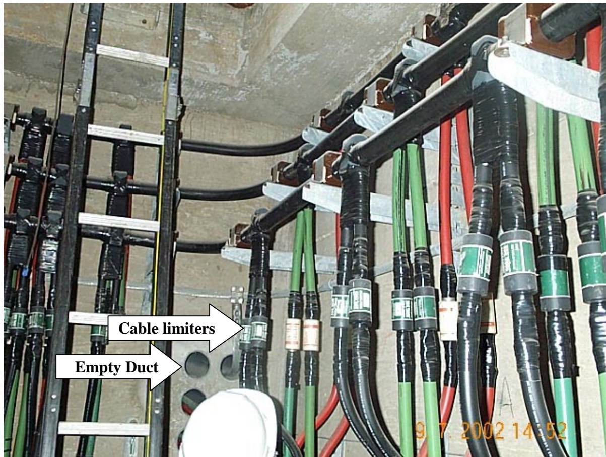
Figure 13 Secondary Bus Hole Showing Quality Workmanship
