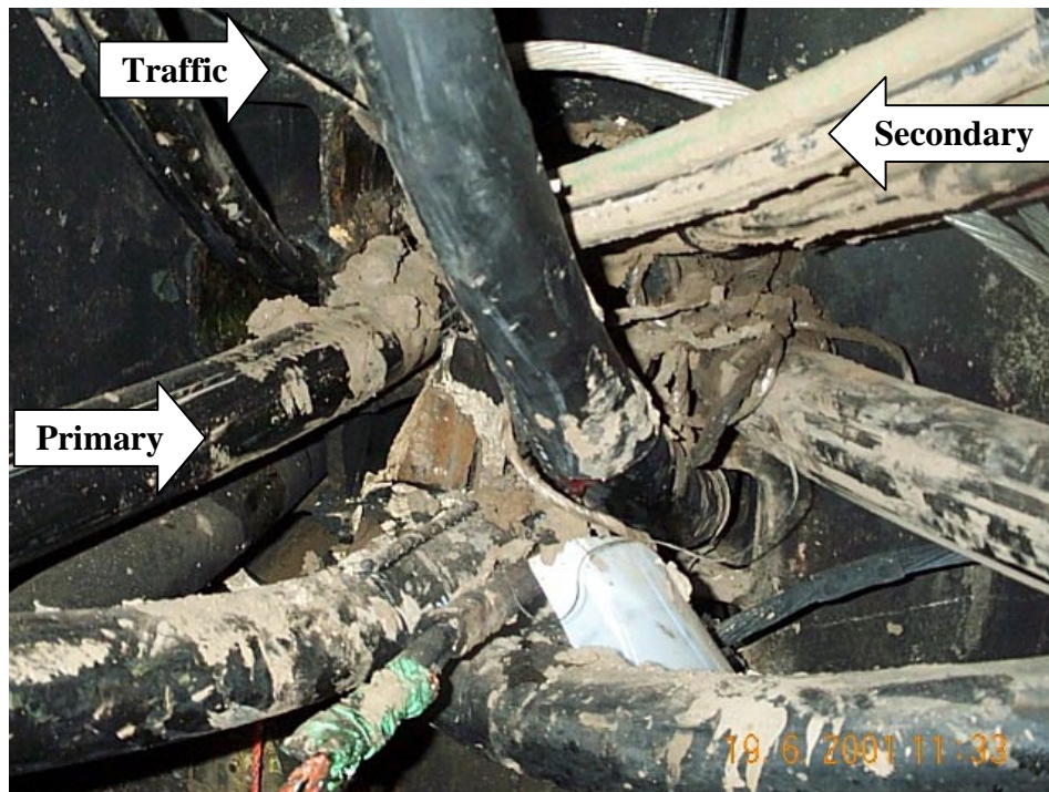
Figure 4 Crowded Manhole within Georgetown with Primary Cables, Secondary Cables, and Traffic Signal or Street Light Cable
