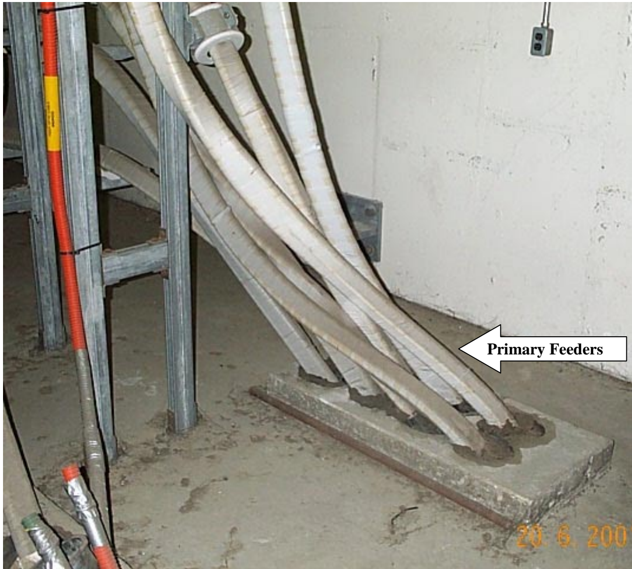
Figure 22 Primary Feeders in Substation Showing Good Workmanship
