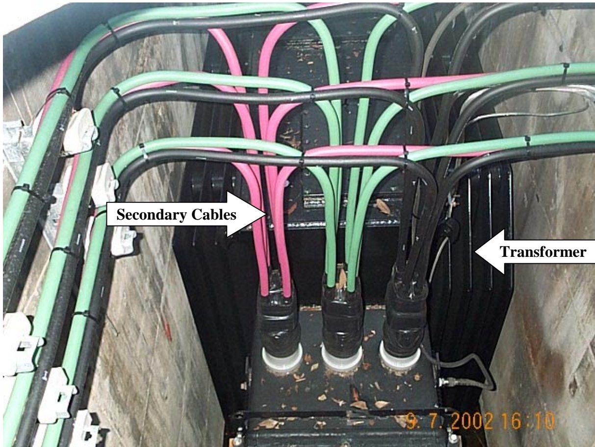
Figure 19 New Transformer Vault with Neatly Arranged Secondary Cables
