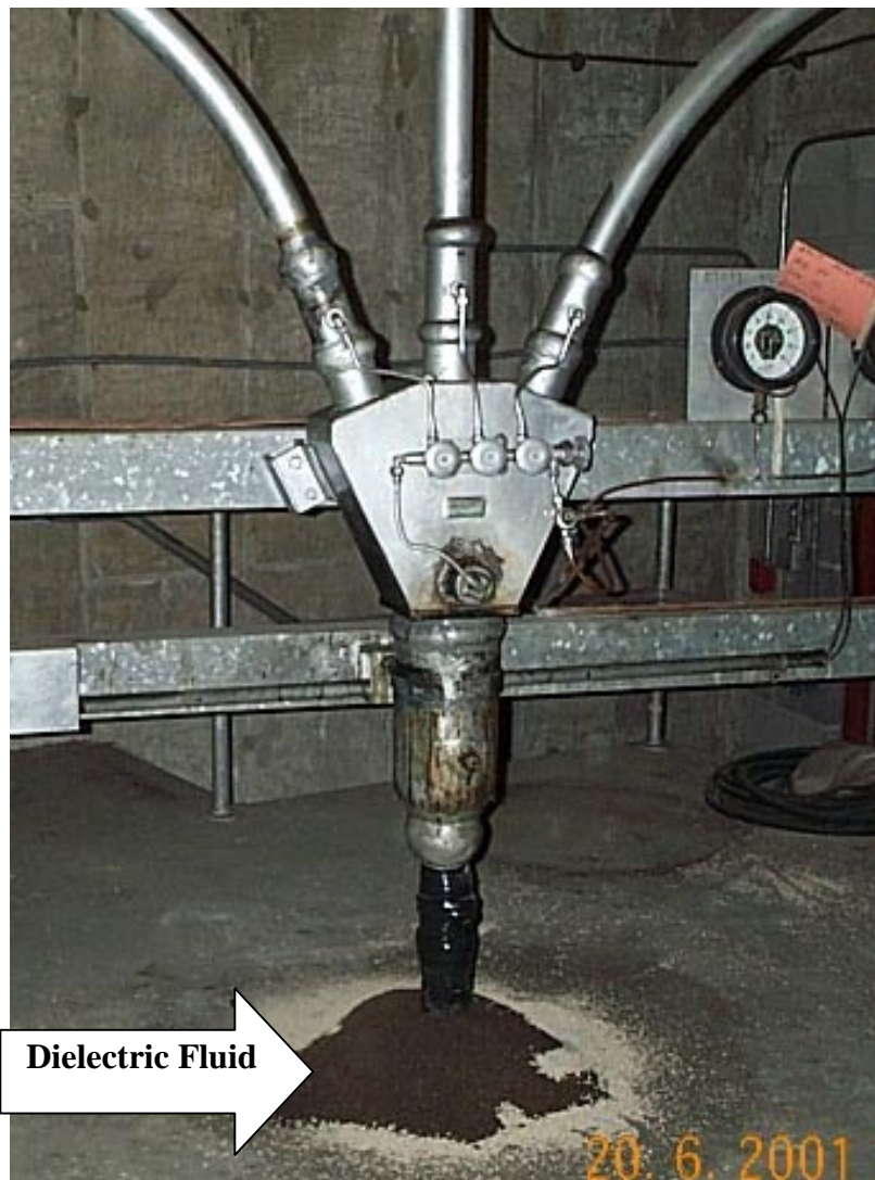
Figure 21 69 kV Transmission Cable Leaking Dielectric Fluid
