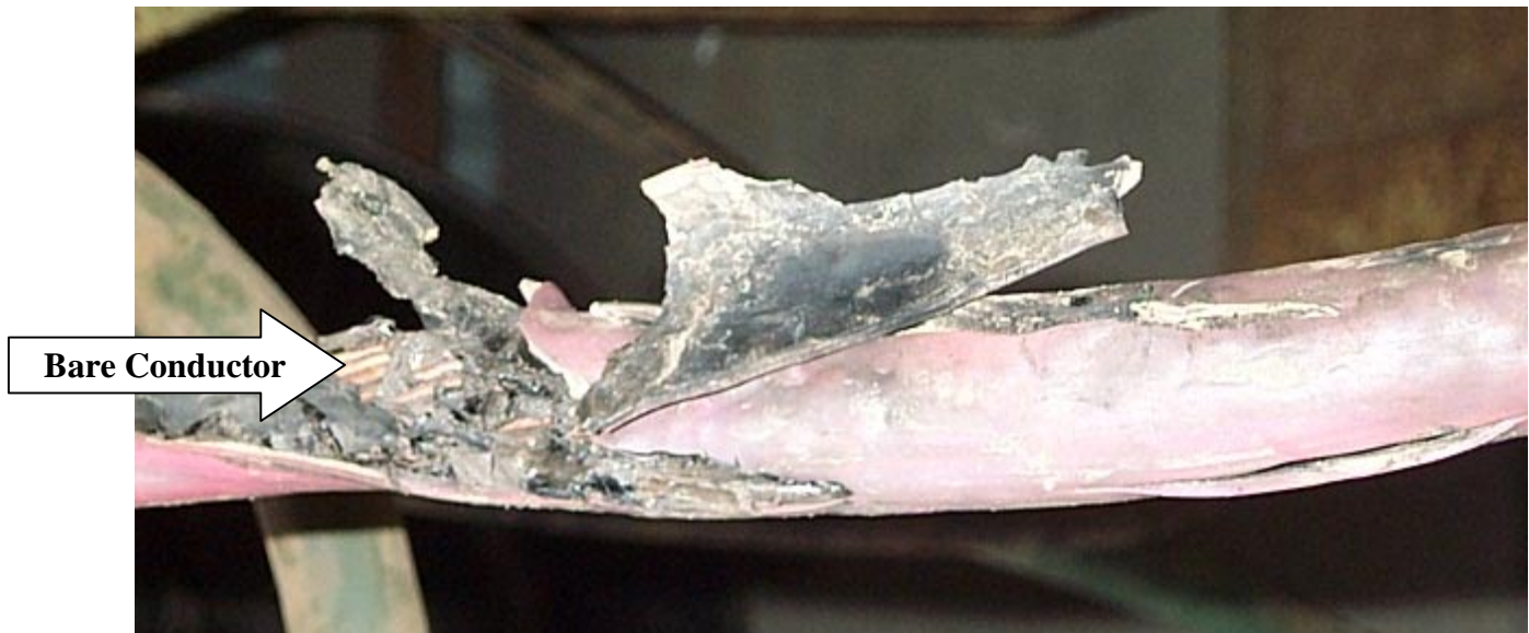
Figure 8 Overheated Secondary Cable Removed from Georgetown after a Manhole Incident
