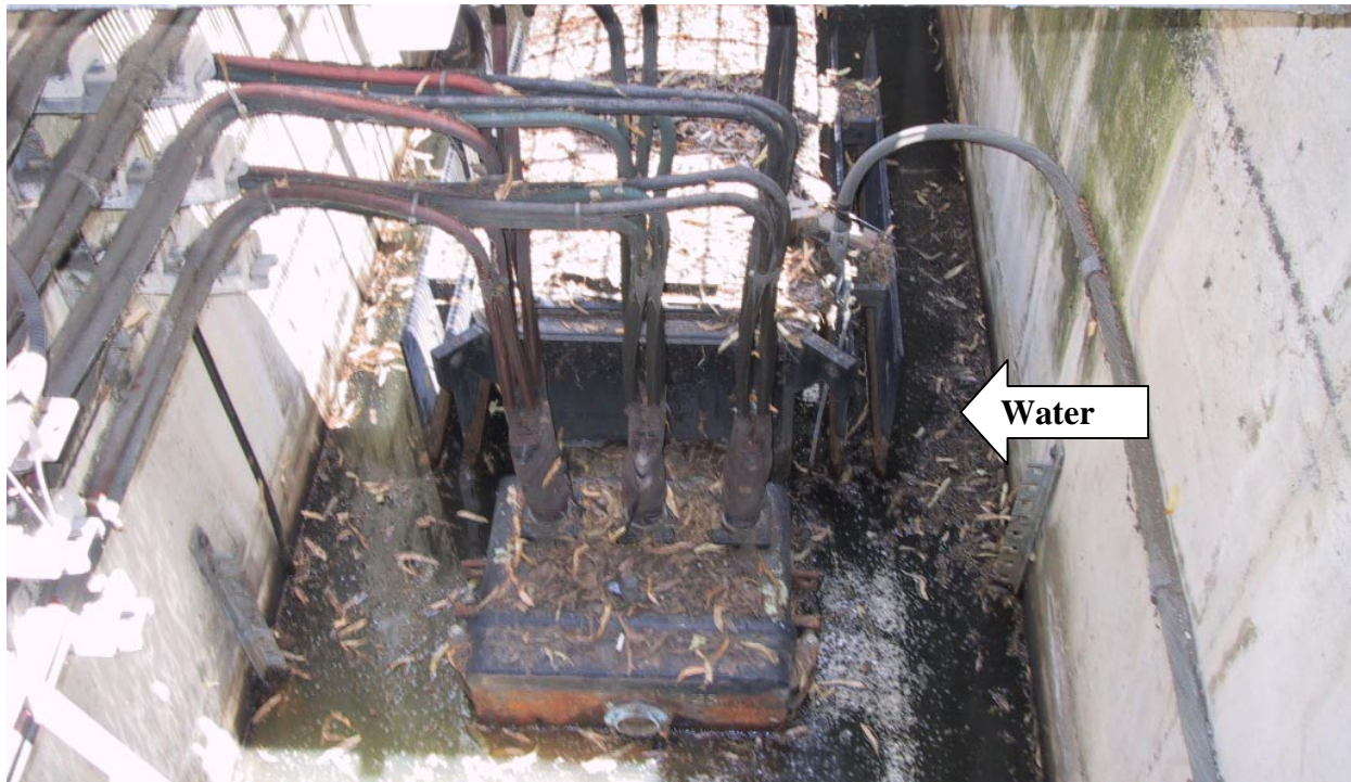
Figure 20 Flooded Transformer Vault with Debris
